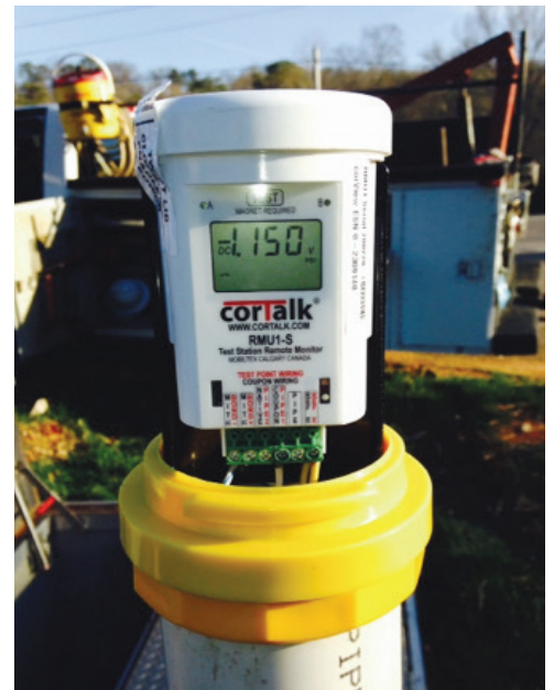
The RMU1 remote monitoring unit from Mobiltex, powered by the Globalstar STX3, shown with test station cover removed monitoring external corrosion protection on an underground pipeline.
